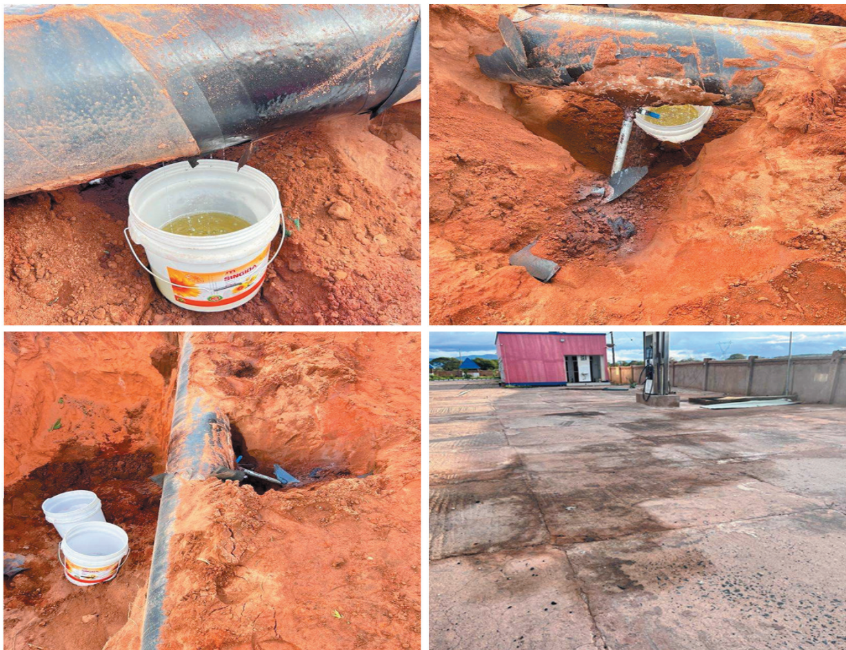
Figure 31: TAZAMA pipeline that was pierced and connected to a one-inch pipe linked to a petroleum storage underground tank of the nearby petroleum retail outlet
